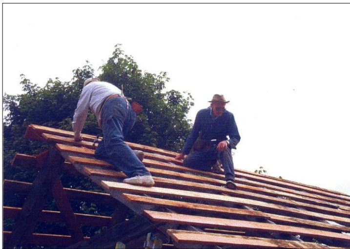
Fig. 35 – Vernon Jenkins, right, and unidentified person installing roof purlins on the Barker Cabin, July 2, 2002. (Courtesy Lynda Jenkins, HSFW.)
