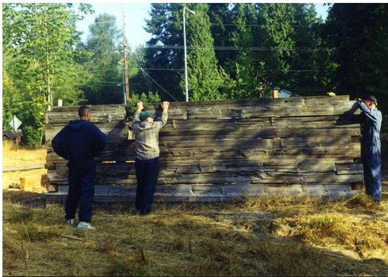
Fig. 27 – Unidentified person, left, Jim Cron, center and Vernon Jenkins replacing the original logs onto the sidewall pen of the Barker Cabin, October, 1999. (Courtesy Lynda Jenkins, HSFW.)
