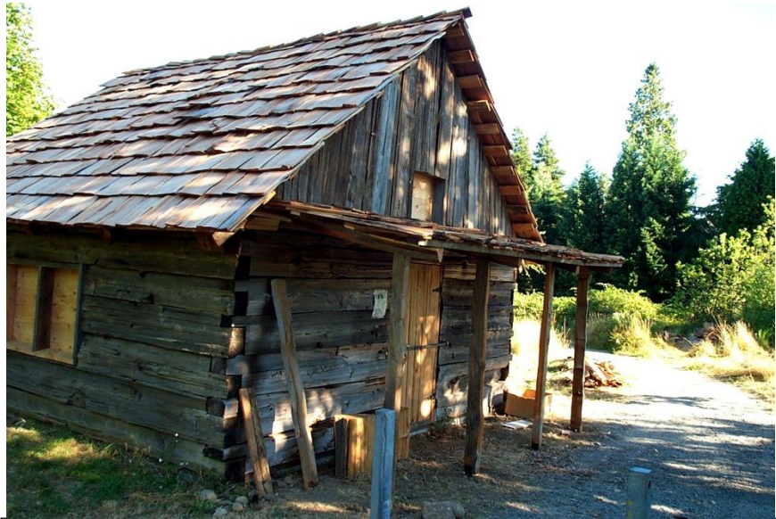
Fig. 38 – The Barker Cabin when essentially restored, after roof construction but before window installation, August, 2002. (Courtesy HSFW.)
