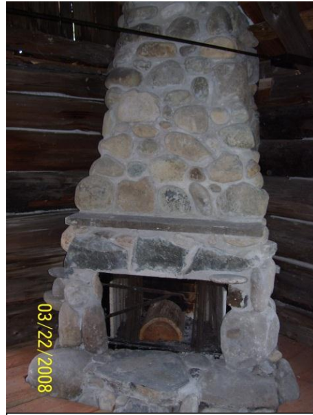
Fig. 44 – The restored fireplace and chimney in the Barker Cabin, March 22, 2008. (Courtesy HSFV.)
