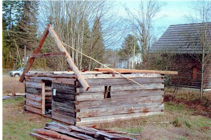
Fig. 32 – Barker Cabin showing the start of its roof replacement, July 2001. (Courtesy HSFW.)
