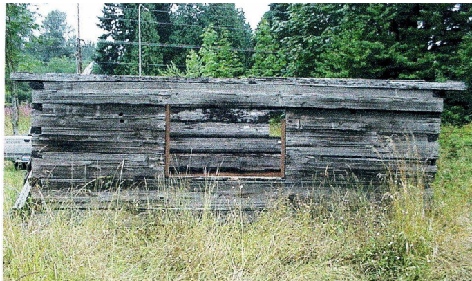
Fig 20 – Temporary reassembly of sidewalls, with the large double window opening on the south side of the cabin, Circa mid 1990s. (Courtesy HSFW.)
