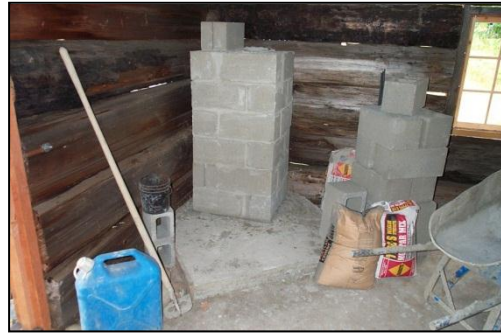
Fig. 41 – Preparing to install the fireplace in the Barker Cabin, 2008. (Courtesy of HSFW.)
