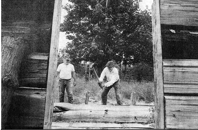
Fig. 31 – Jim Cron and Ed Opstad, with sledge hammer, splitting the cedar log for use on the Barker Cabin restoration, July, 2000. (Courtesy Tacoma News Tribune.)
