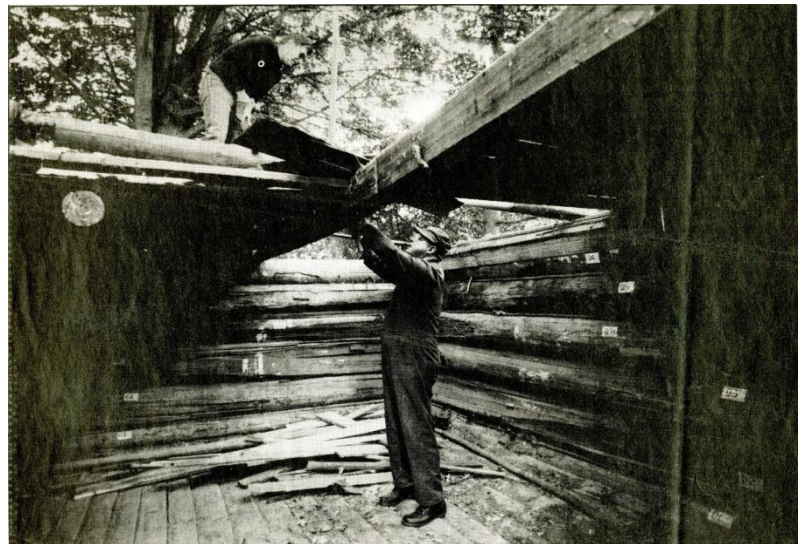
Fig. 16 - Don Miller, bottom, removes nails from the components of the Barker Cabin during disassembly in preparation for the move. On the roof is Doug Pfeffer, President of the HSFW in 1993. (Courtesy Federal Way News .)
